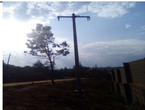
Power supply to Petrocom
