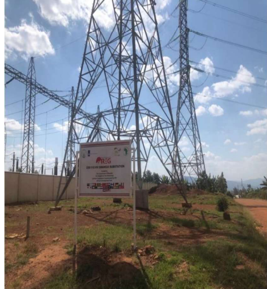
Connection point at Shango substation
