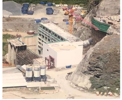
Rusumo HPP-Power house
