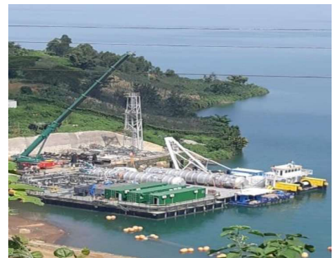
Gaz extraction facility of Shema
