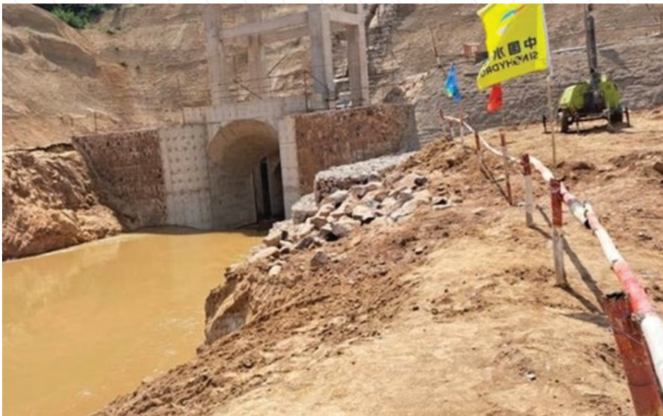
Nyabarongo II Hydroelectric Power Station, with installed generating capacity of 43.5 megawatts
