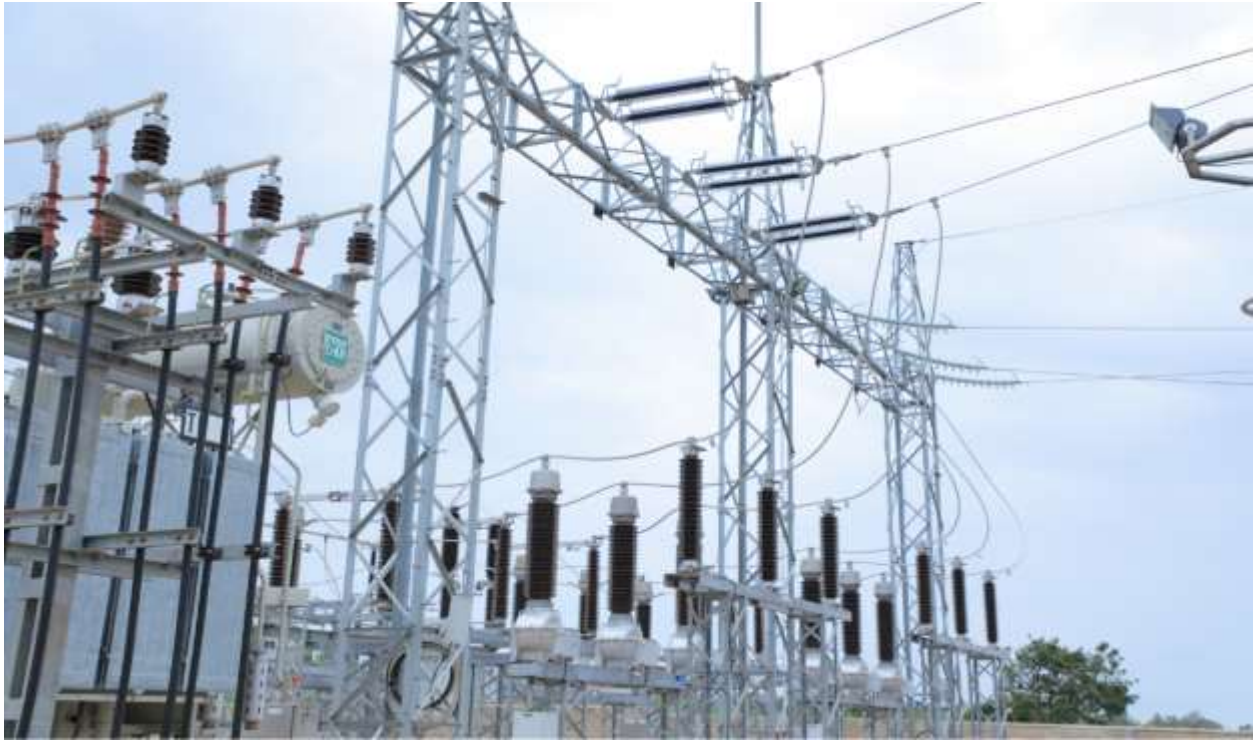
Figure 3: Gahanga substation, completed along Mamba-Rwabusoro-Bugesera-Gahanga line
