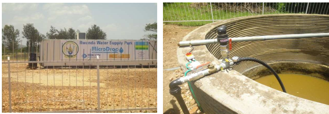
Water treatment plant at Nyabwishongwezi
